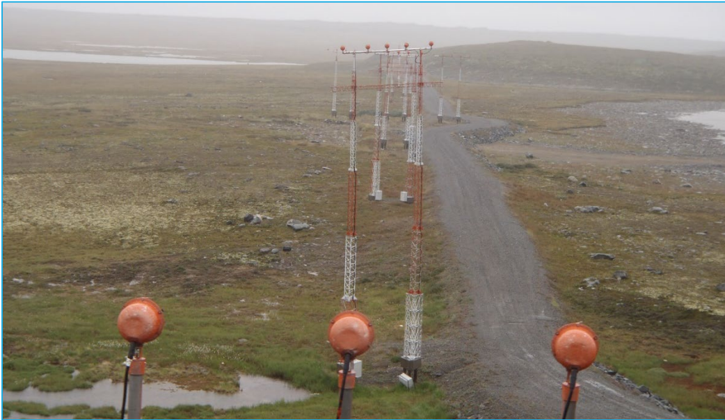
Figure 9.4 - Runway 13 Approach Lighting Rankin Inlet Airport (2010)
