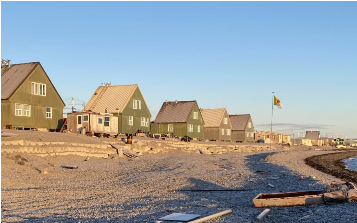
Figure 2-18 Damaged concrete block seawall in front of houses #105 to #110 (2021)
