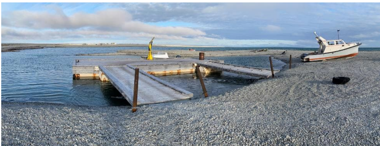
Figure 2-4 Sanirajak floating dock
