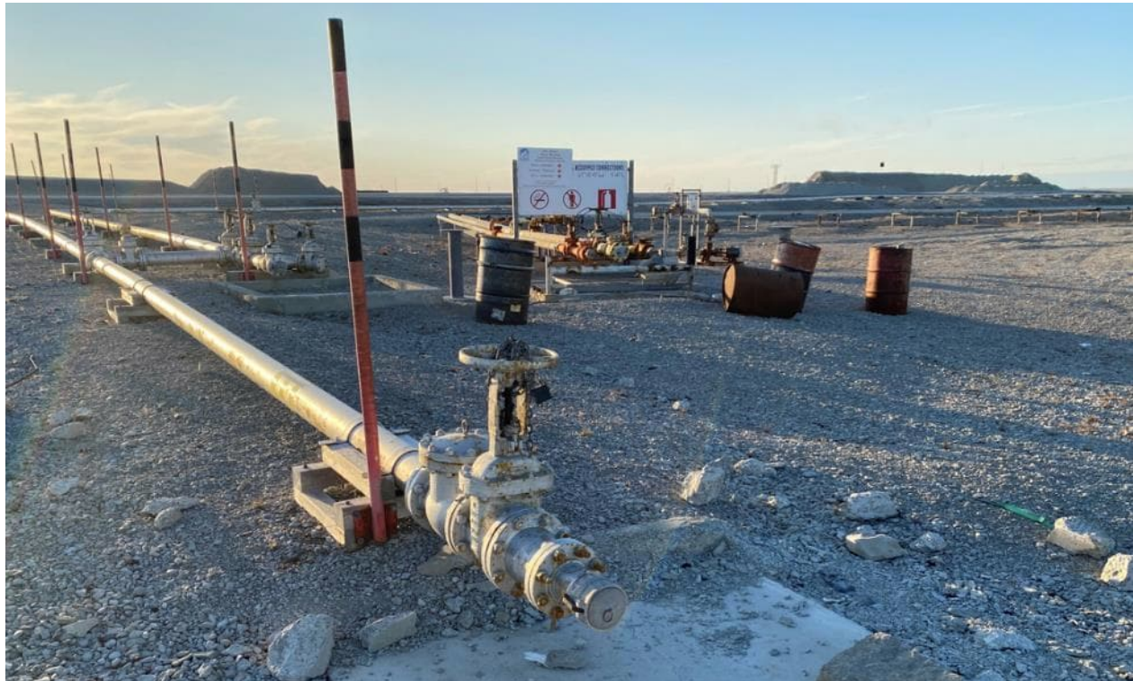
Figure 2-6 Sanirajak fuel manifolds
